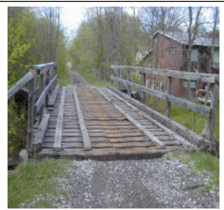
Fig 3: Timber on surface of bridge
